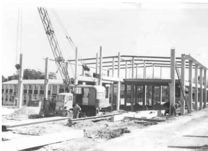
Construction continued during the School's 2nd year, 1961. E block, foreground with TAS Block (Industrial Arts) in the background.
