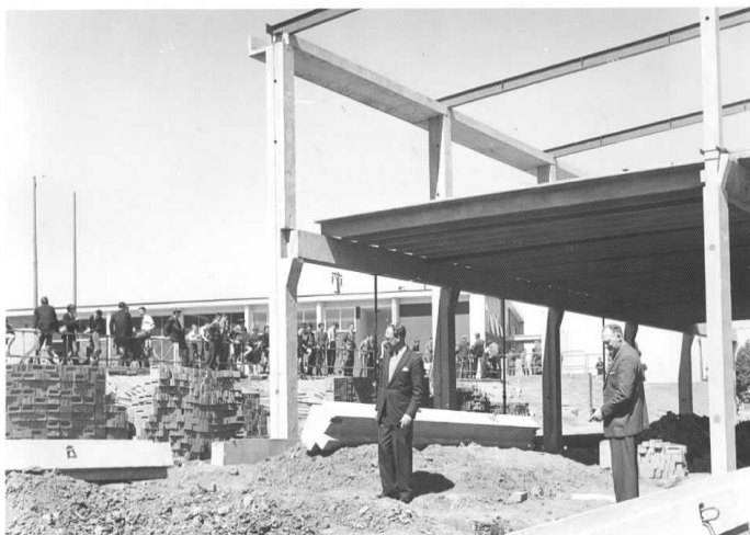
Deputy Principal, John Holme (left) with Principal Mervyn Brown, inspect progress of E block during construction in 1961.
